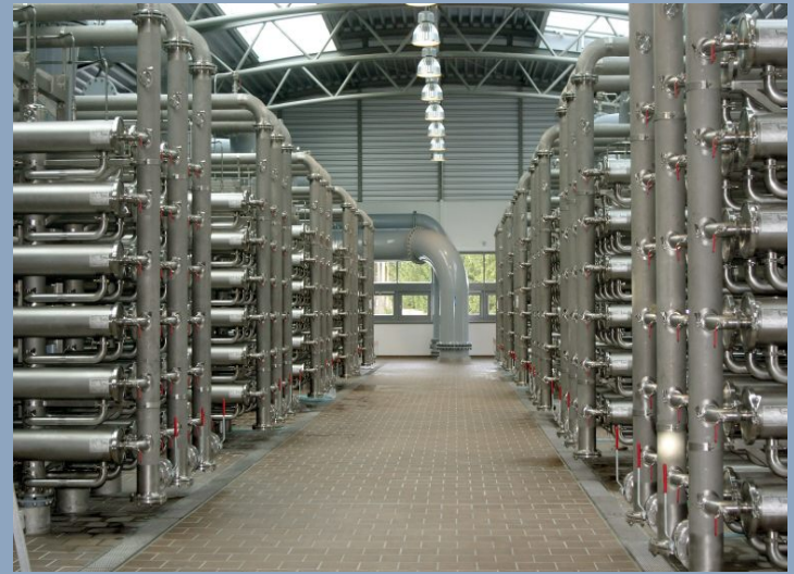
UF Water treatment plant Roetgen ENWOR, Germany © ENWOR
